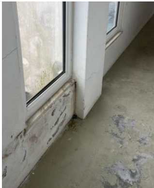
Green Stains and efflorescence
