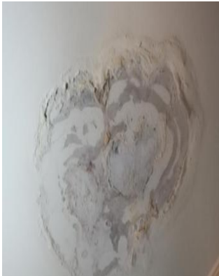
Efflorescence and detachments
