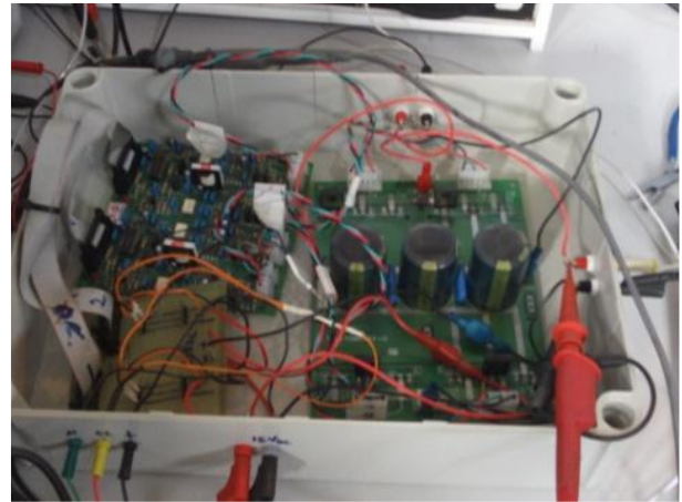
Fig. 17: Power circuit with a driver that serves as an interface between the power source and the motor.
