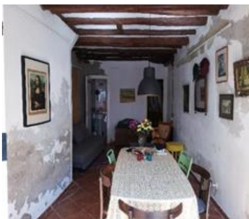
Fig. 2 Manifestations of pathologies in part due to inadequate ventilation, and other causes identified through the model.
